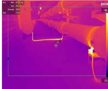
FIG. V-11. Main Transformer A GIB Ground Wire.
