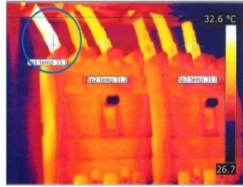
FIG. V-8. Main Transformer Phase C Control Panel.
